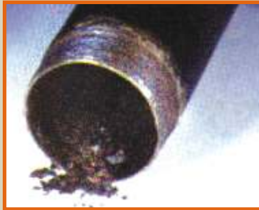
Real life problem 2 Corrosion of Piping
